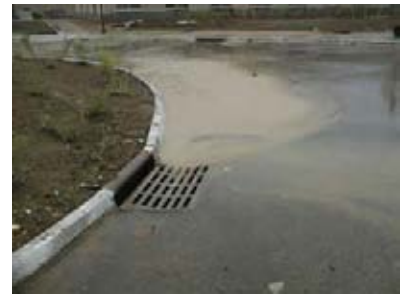
Sediment-laden water entering a storm sewer
